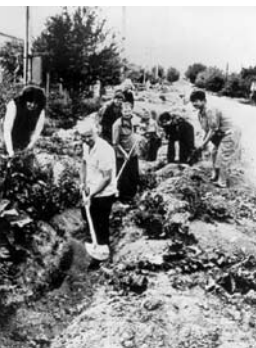
Figure 6: Residents of Sevastyanovka participate in excavation work for the water distribution network
