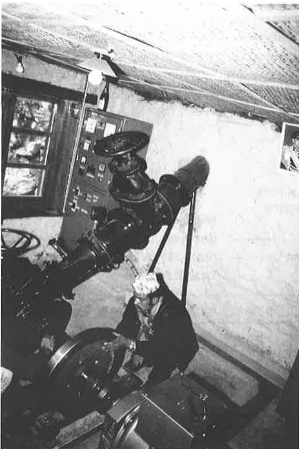
Photo 3: Namche Bazar (Category A) Electro-mechanical equipment
