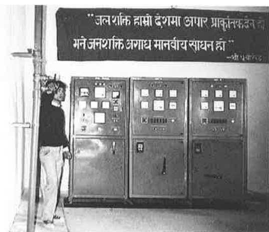
Photo 3: Syangja power plant (Category C) Control and synchronisation panel
