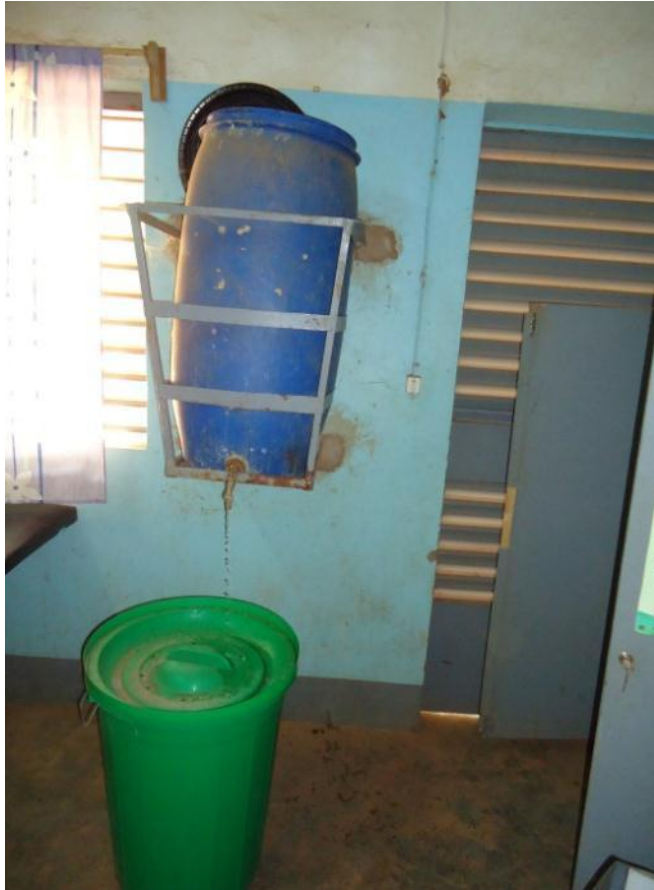
Water supply in a health center in Burkina Faso
