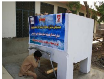
Provision of drinking water outside HF
